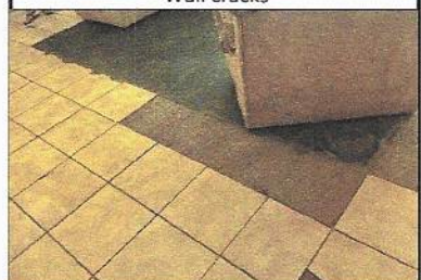
Some missing floor tiles
